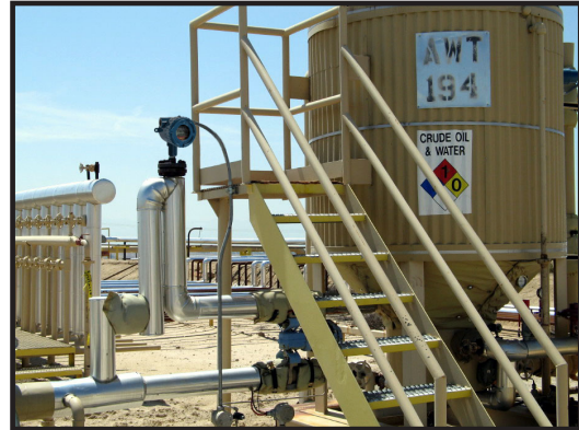
Drexelbrook installation coming off the AWT and then fed back to the manifold.
